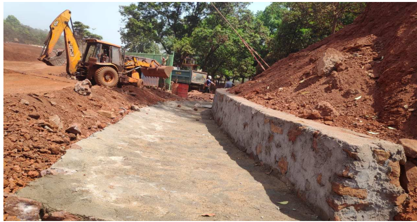
Photo showing siltation cum percolation pond and garland drain
